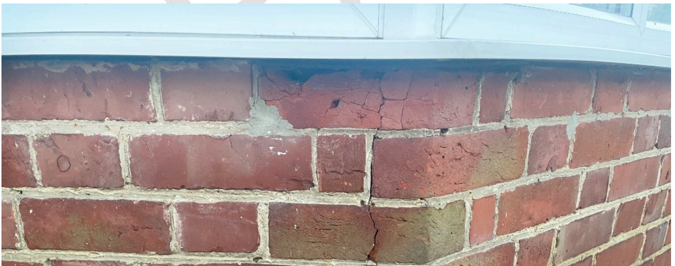
Squints are cracked due to baypole pressure
